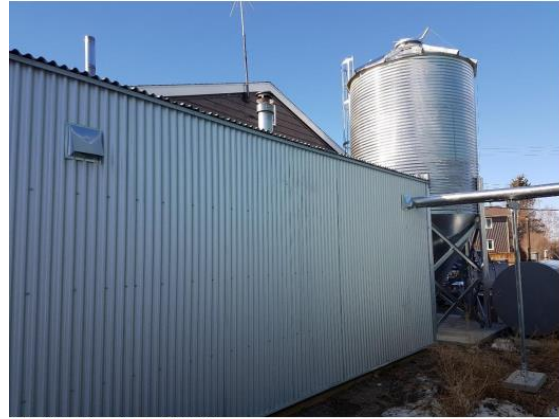
Photo 1: New Energy Box and Pellet Silo
