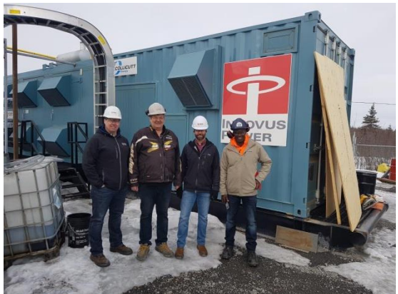
600 kW Variable-Speed Generator - Aklavik (2018)
