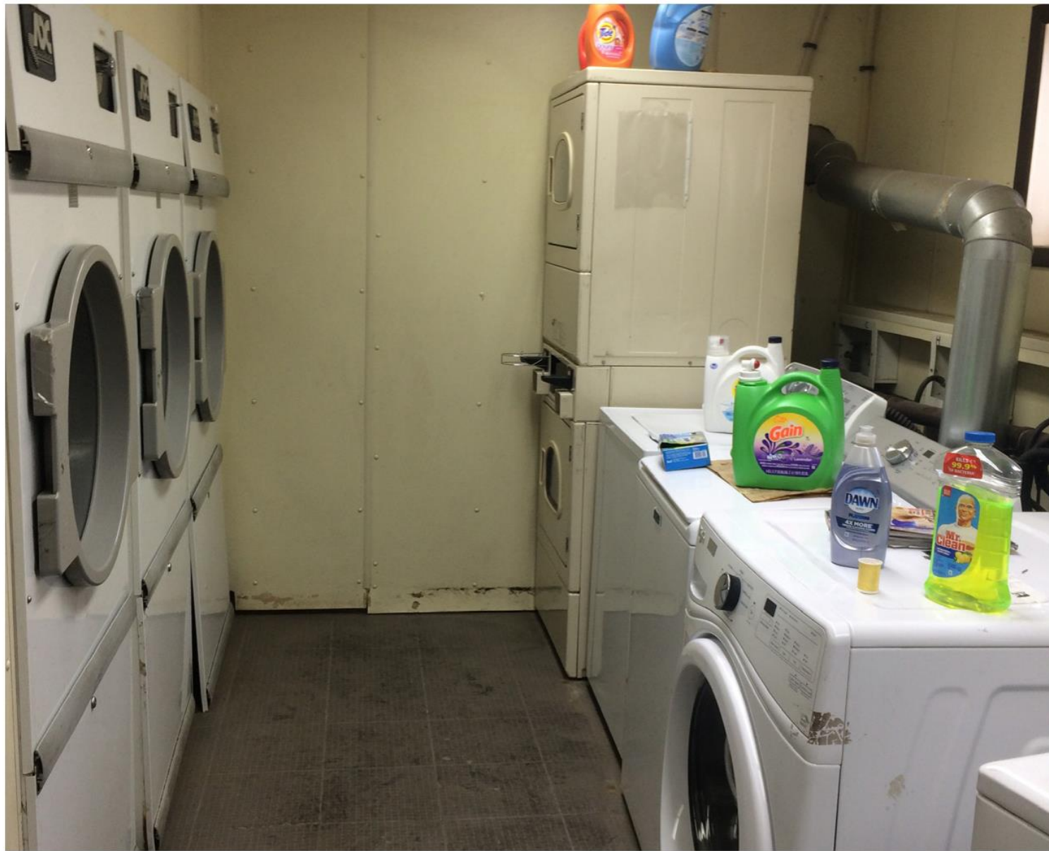
Above: Two functioning washers and two functioning dryers are shared between 400 people at Kivalina's washeteria.
